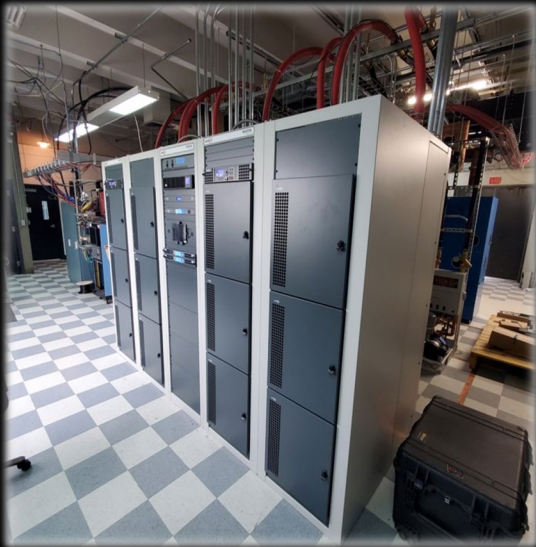
75kW Average Power in <math>\frac{1}{2}</math> the space as a Tube System
